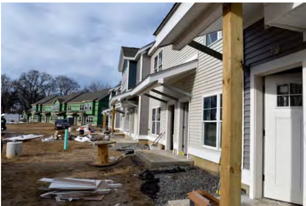
A view of Rosewood Way Townhomes, Way Finder's new affordable and market-rate housing development in Agawam. (Don Treeger / The Republican) The Republican
