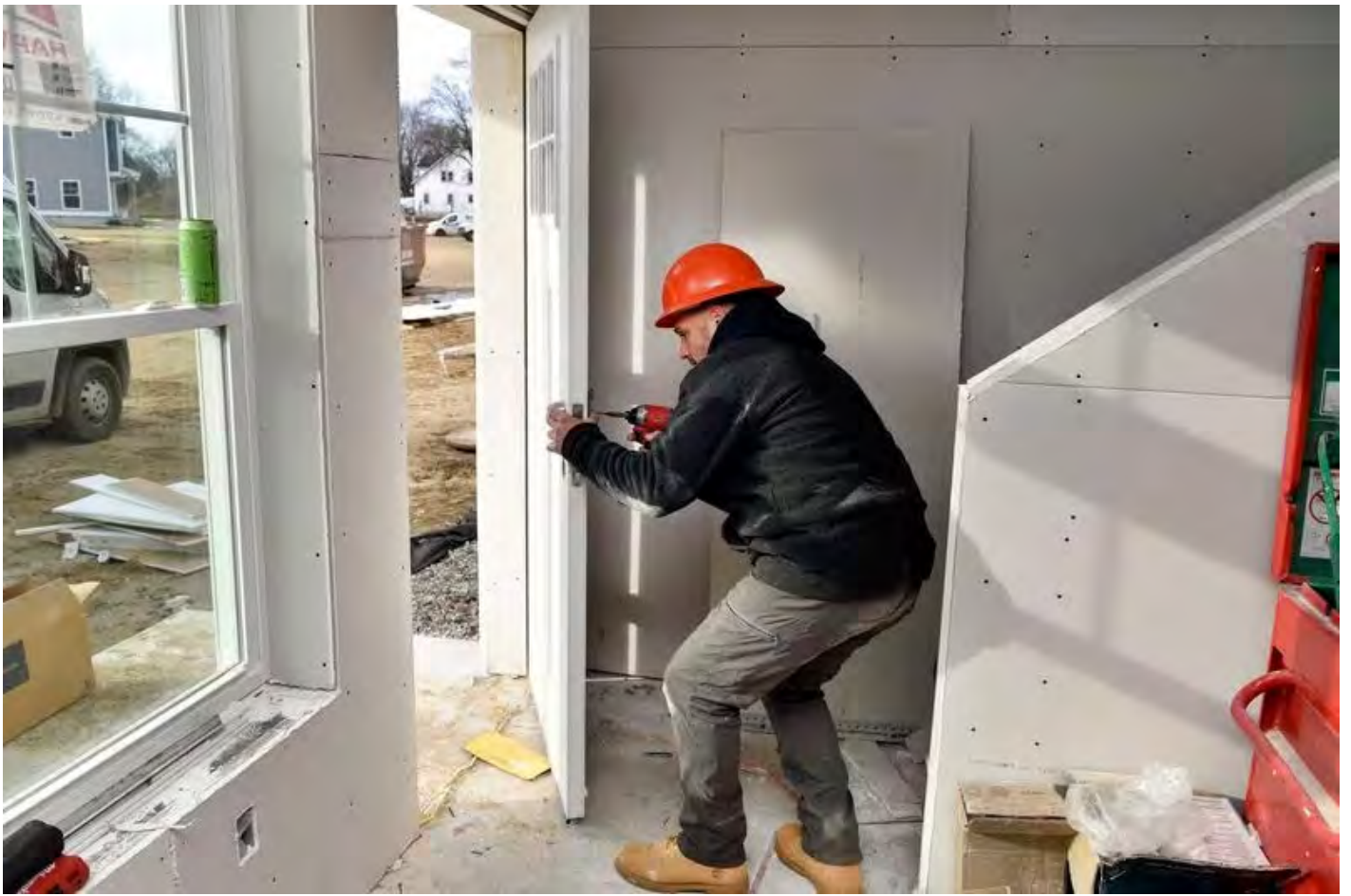
Above: Carpenter Paul Pennell of Holyoke installs door hardware on a unit at Rosewood Way. (Don Treeger / The Republican) The Republican
